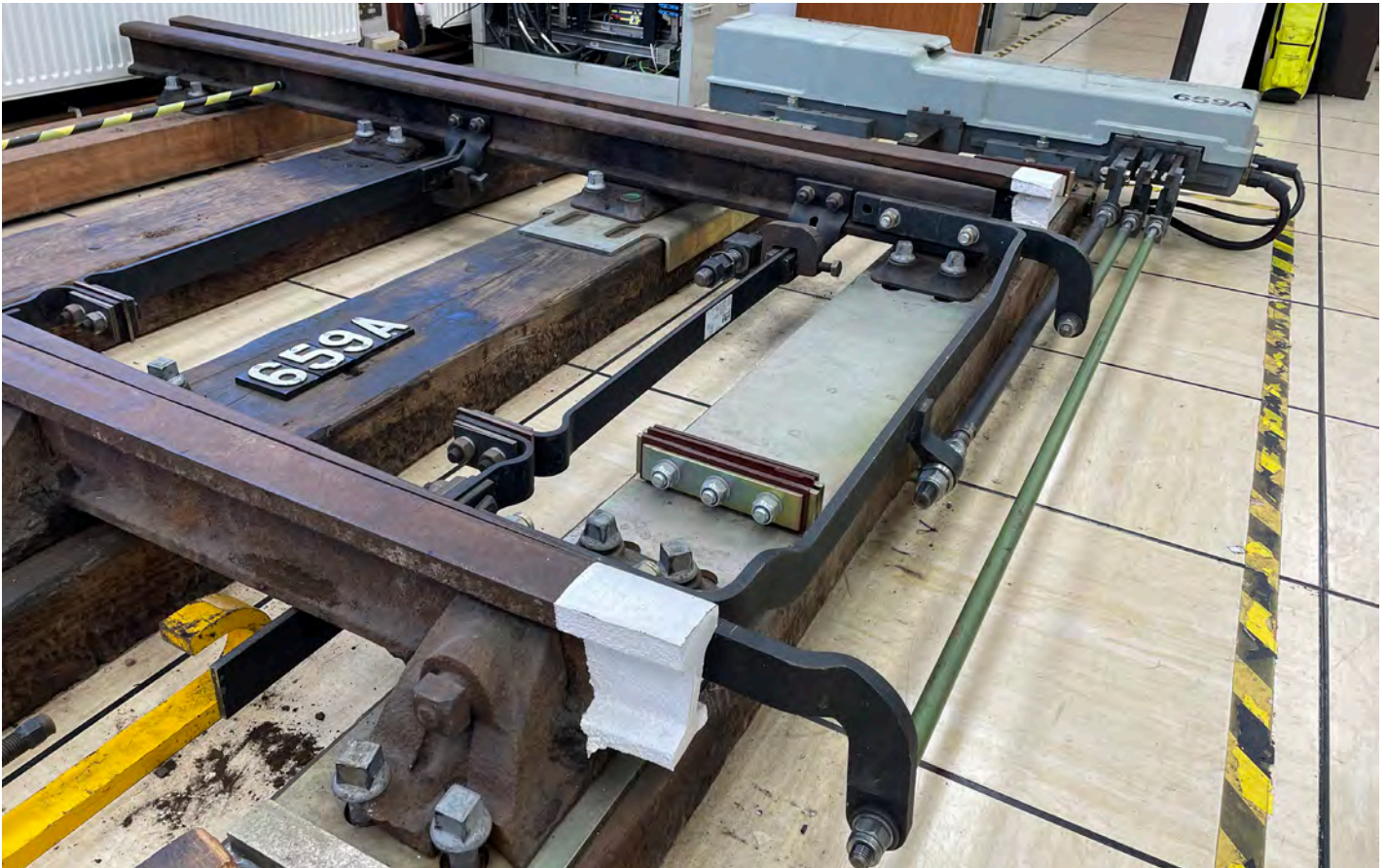
Figure 8 – A typical point machine arrangement (in a training school environment) showing the drive rod, detection, FPL rodding connections, and associated stretcher bars. Image Trevor Bradbeer and Signet Solutions.
