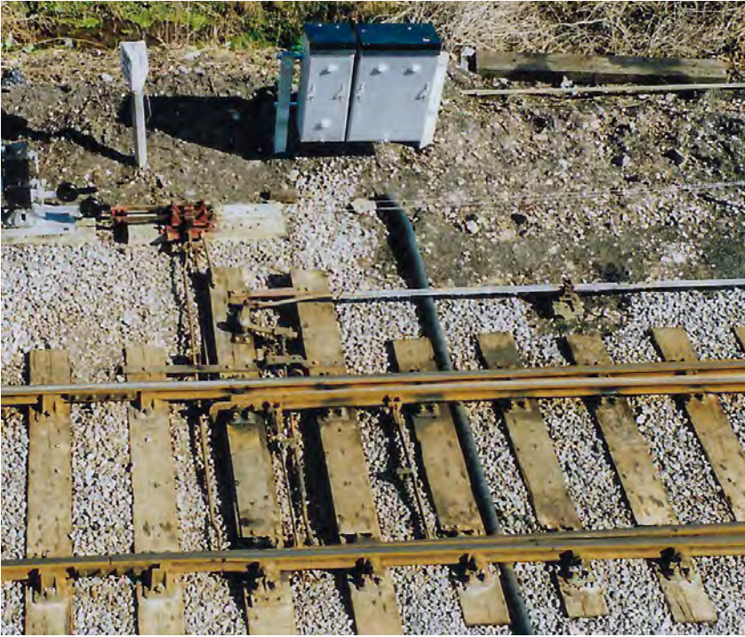
Figure 5 – Points rodding leading from the signal box (out of picture, to the right) to a set of points, with cranks that are used to transmit the motion of the rods through a right-angle. Photo John Francis.
