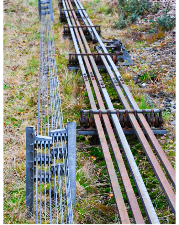
Figure 6 – Close-up of a rodding run for several sets of points (a wire run for signals is on the left). Photo Ian J Allison.
